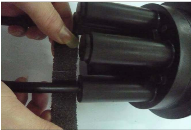
(10) Sand the cable and entry ports that need to heat-shrink by abrasive paper. Wipe the dust that be left after sanding away.
