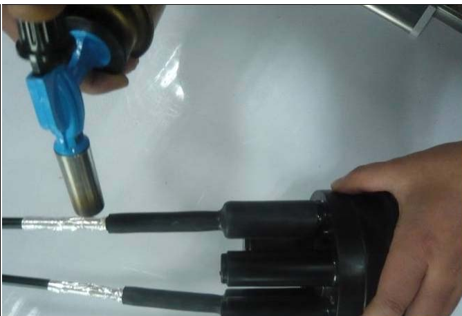
(12) Put the heat-shrinkable tube on the entry ports, then heating by blast burner and stop heating after it is tighten. Let it be cool naturally.
