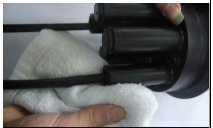
(9) Sealing of the cable and the base: clean the entry ports and cable with 10cm long by scrubber
